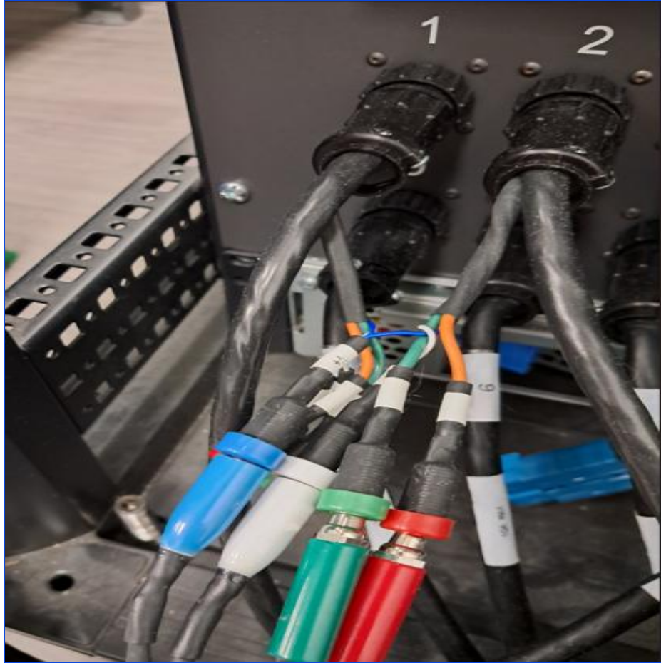
Figure 64: Gamry Connectors plugged into UHPC Channel Cable
